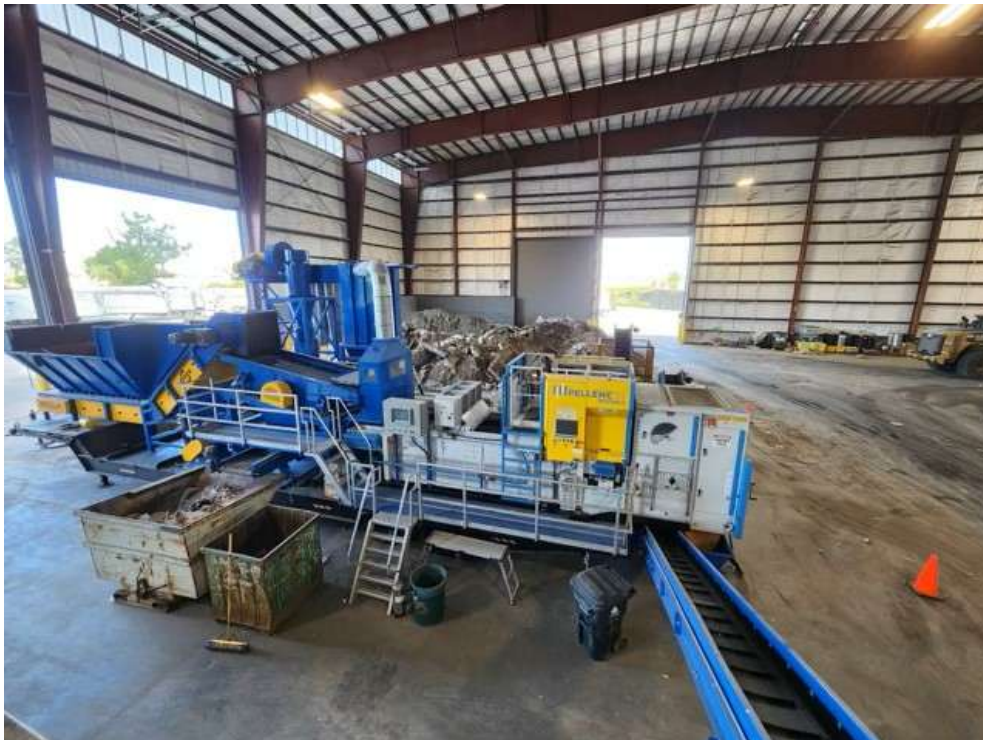
Figure 8 - Portable Secondary MRF System
